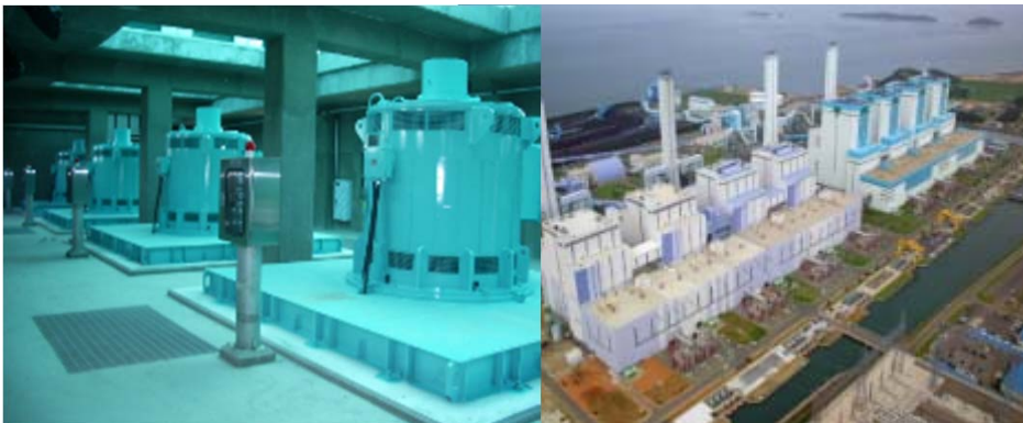
Intake Pumping Station for Circulating Water System of Boryeong TPP #7,8
