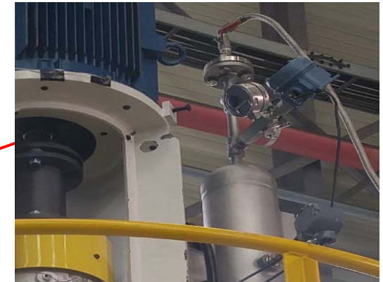
[Press/Level of Reservoir] Alarm display for mechanical Seal is damaged
