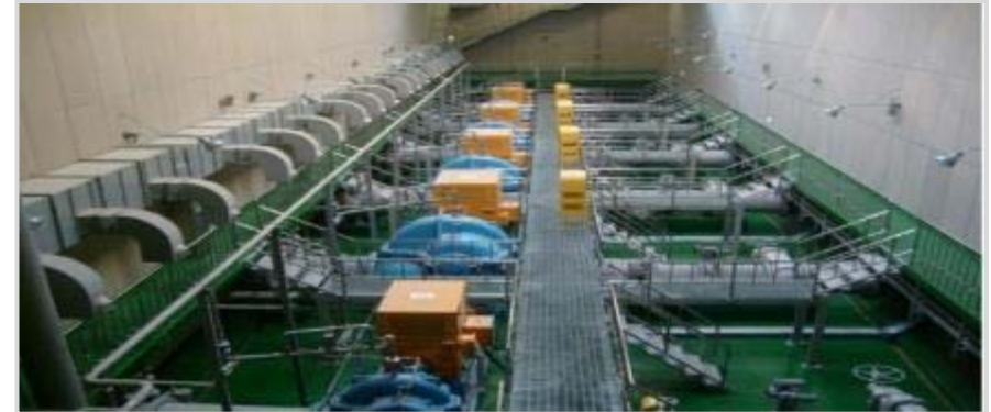
Gu Eui - Jayang Pumping Station
