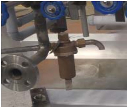
[Safety V/V] Liquefied nitrogen Tank (10bar)
