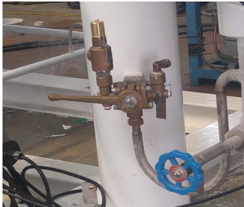
[Safety V/V] Pump test Chamber (4bar)
