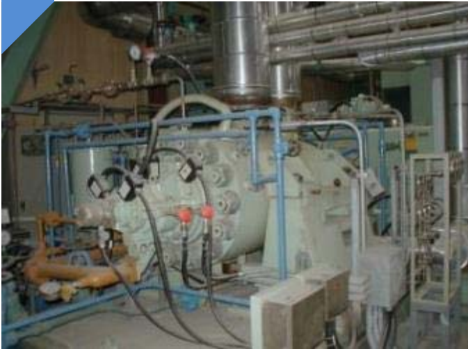
Tangjin TPP #1~4 PJT (500MW)
