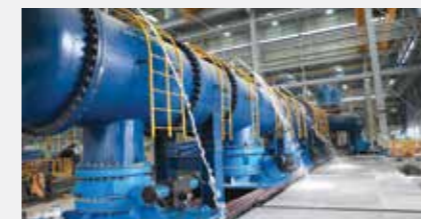
Large Capacity Pump Test Facility
